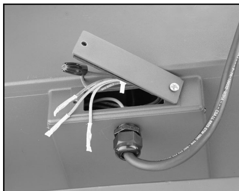
VOLTAGE TAP COMPARTMENT
